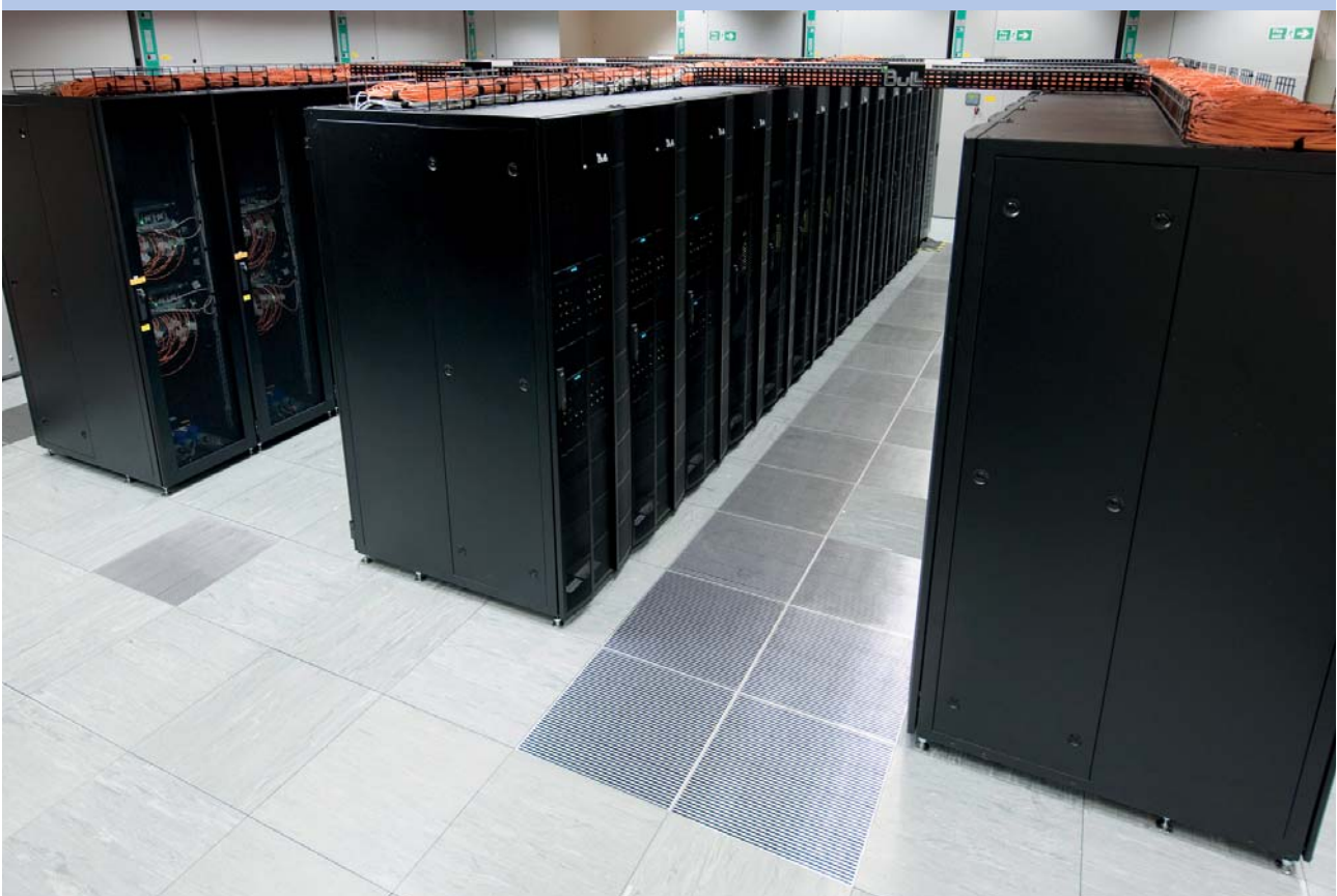
The Bull capability computer, Blackthorn, installed at AWE.
