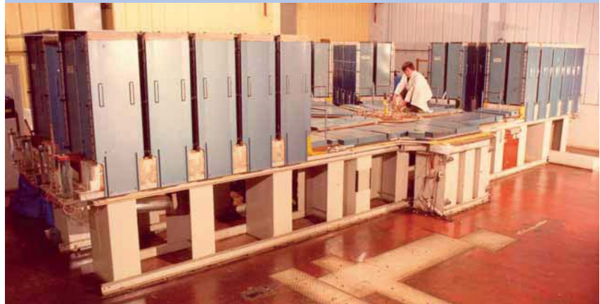
GRIMM capacitor bank.
